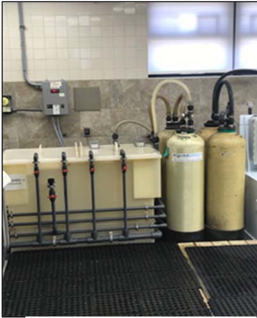
Part of an Ion Exchange System at a Permitted Zero Discharge Facility
