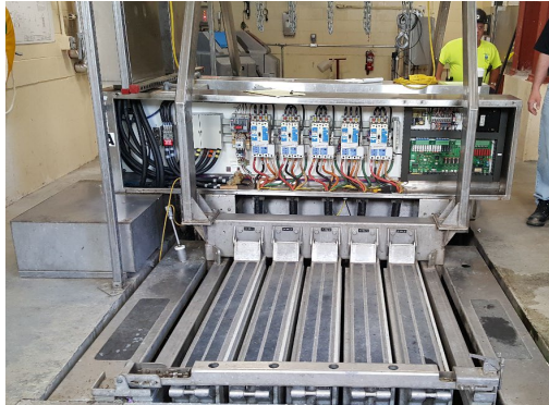
Photo: Bucklin Point UV Disinfection System
