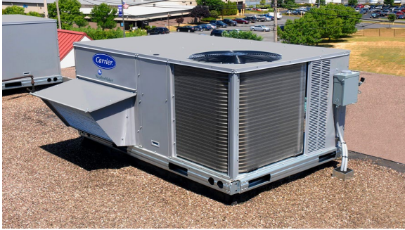
Photo: Carrier Rooftop Air Conditioner
