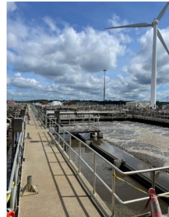
Field's Point Aeration Tank
