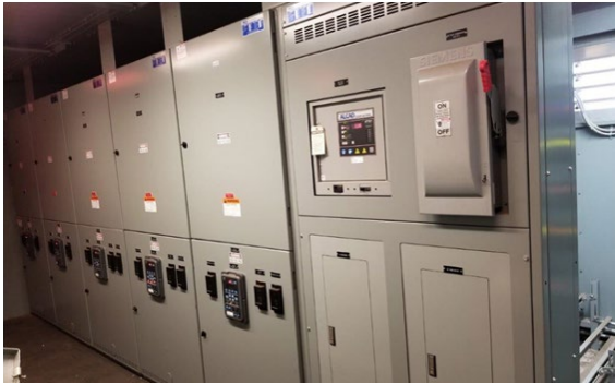
Photo: Field's Point Electrical Facility
