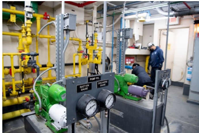
NBC Mechanics repairing valve in the Sodium Hypochlorite Building Photo by Peter Goldberg
