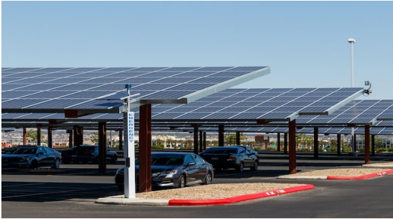
Photo: Solar Carport
