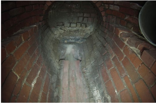
Photo: OF 056 Regulator on Vandewater Street
