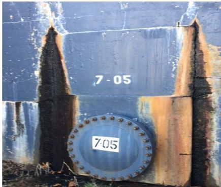
Photo: Secondary Digester
