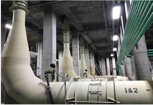
Photo: CSO Tunnel Pump Station
