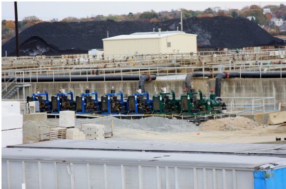
Photo: Aeration Tank Pumps
