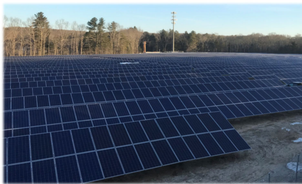
NBC's Solar PPA Facilities in North Kingstown, RI
