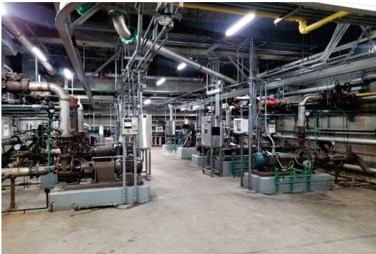
Photo: Primary Sludge Pump Station
