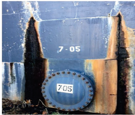
Photo: Secondary Digester
