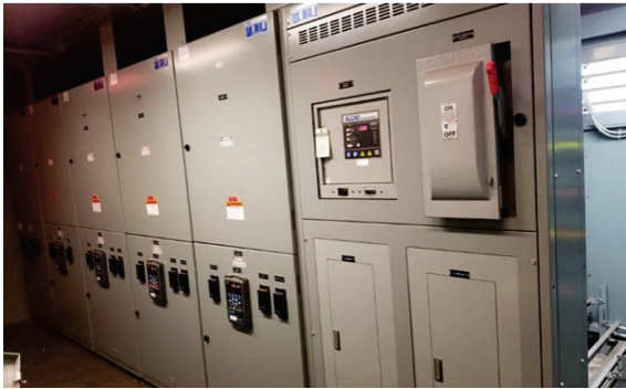
Photo: Field's Point Electrical Facility
