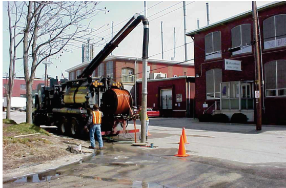
Photo: Interceptor Grit Removal
