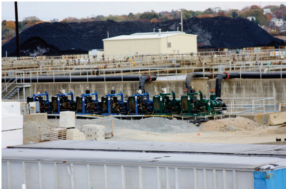
Photo: Aeration Tank Pumps
