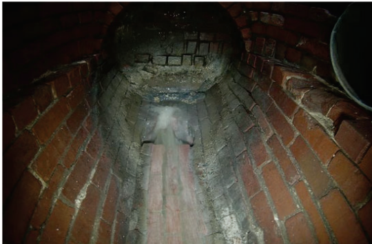
Photo: OF 056 Regulator on Vandewater Street
