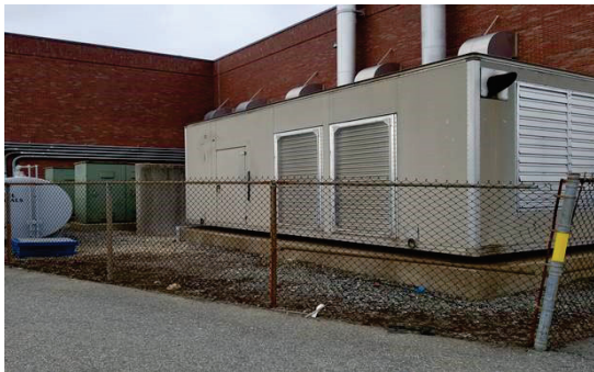
Photo: Field's Point Screw and Blower Generator
