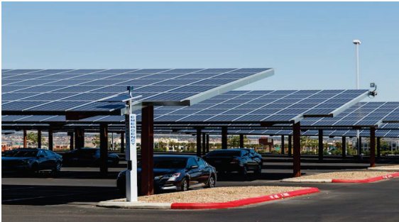
Photo: Solar Carport
