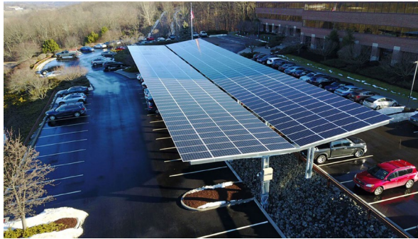
Photo: Solar Carport
