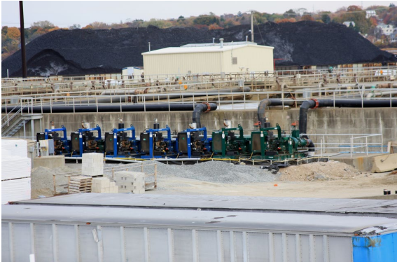
Photo: Aeration Tank Pumps
