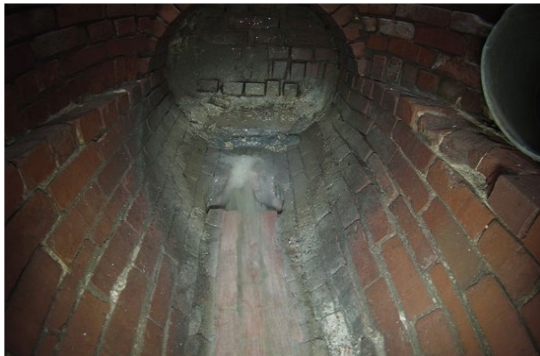
Photo: OF 056 Regulator on Vandewater Street
