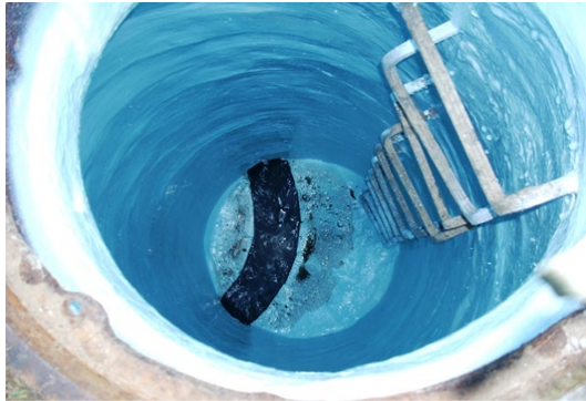
Photo: Flow Monitor
