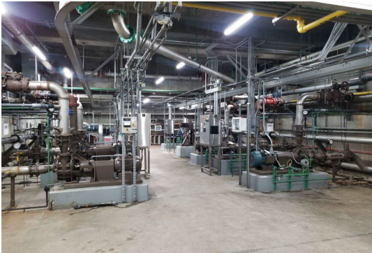
Photo: Primary Sludge Pump Station
