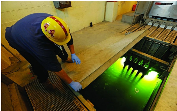
Photo: Bucklin Point UV Disinfection System
