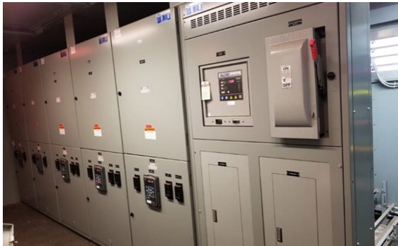
Photo: Field's Point Electrical Facility
