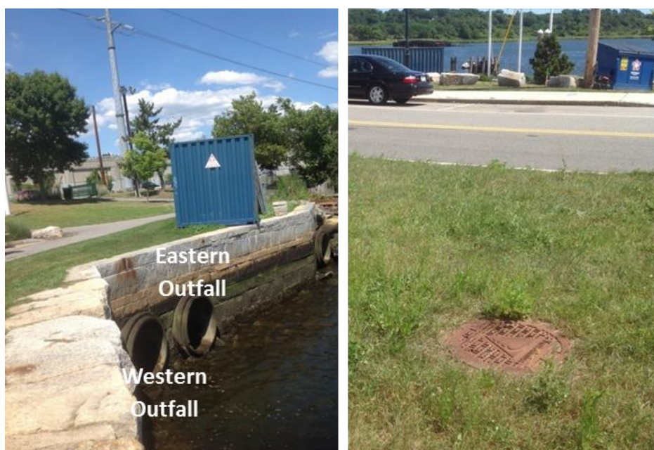
Figure 16. Photographs showing the eastern and western stormwater outfalls, as well as the Vortechinics manhole cover just upstream of the outfalls.
