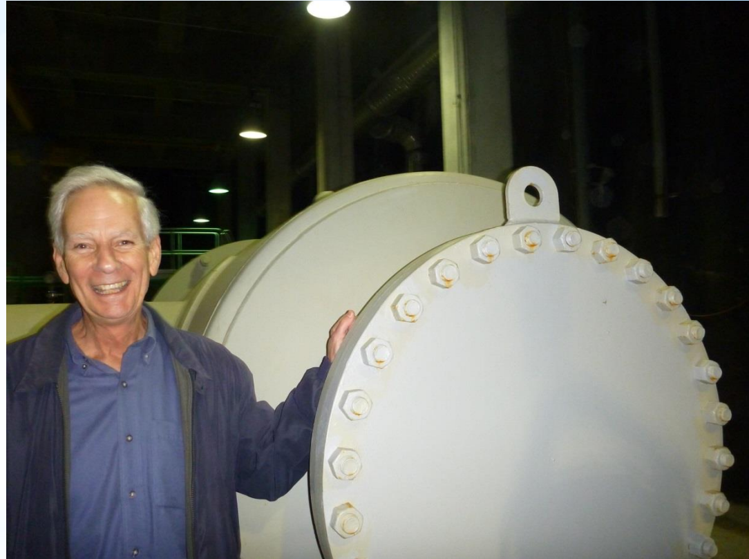
Professor Scott Nixon touring the NBC CSO Tunnel Pump Station
