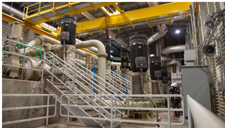
Pump Cavern in CSO Tunnel Pumping Station Photo by Peter Goldberg
