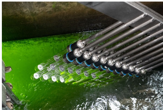
Ultraviolet Disinfection Module at Bucklin Point Photo by Peter Goldberg
