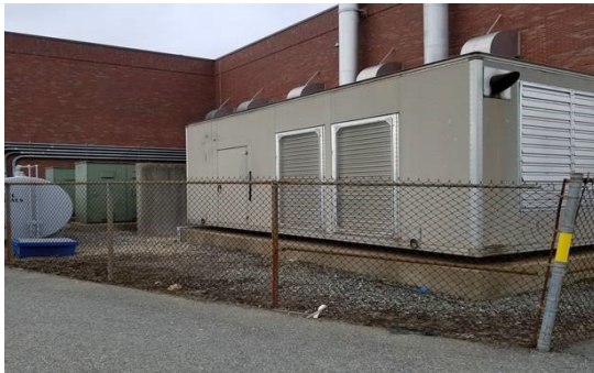
Photo: Field's Point Screw and Blower Generator
