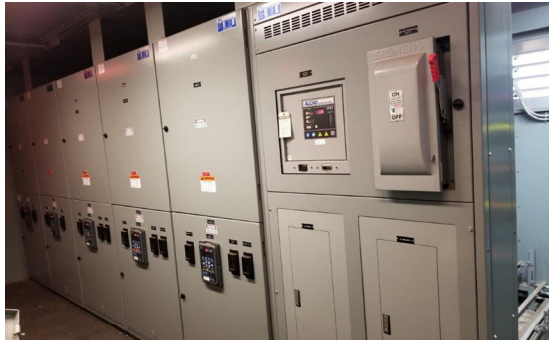
Photo: Field's Point Electrical Facility
