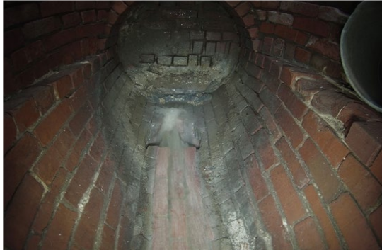
Photo: OF 056 Regulator on Vandewater Street
