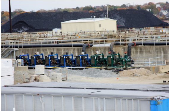
Photo: Aeration Tank Pumps
