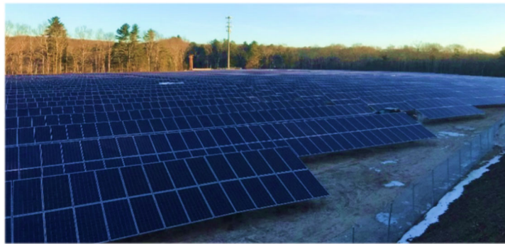
NBC'S Solar PPA Facilities North Kingstown, RI
