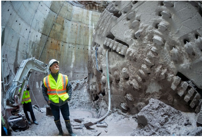
Chairman Mesolella in Front of the Tunnel Boring Machine Subsequent to the Tunnel Breakthrough on February 15, 2024 Photo by Peter Goldberg
