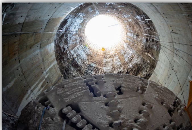
View of CSO Phase III A Receiving Shaft and Tunnel Boring Machine Photo by Peter Goldberg
