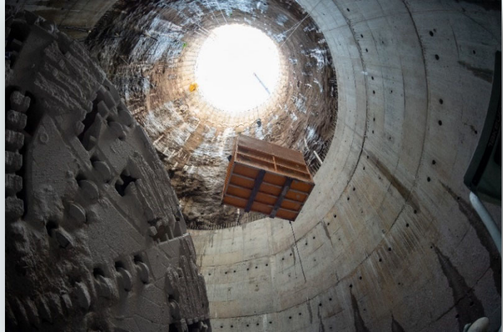
View of CSO Phase III A Receiving Shaft and Tunnel Boring Machine
