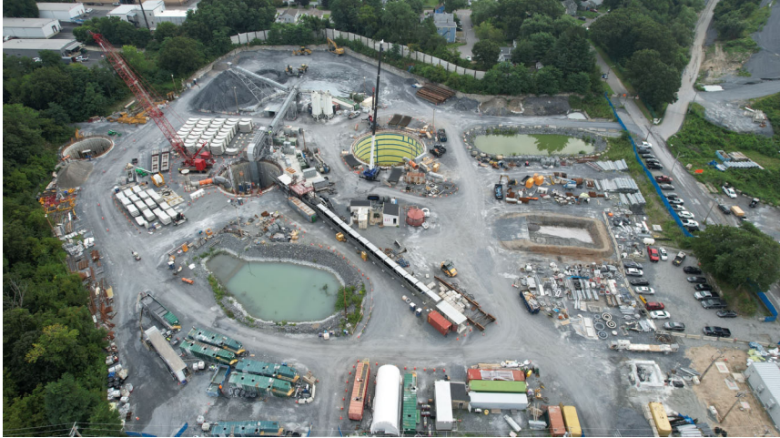
CSO Phase III A Pawtucket Tunnel and Pump Station Shaft Construction Site
