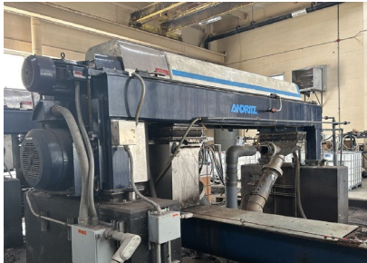
Photo: Centrifuge at Bucklin Point Dewatering Facility
