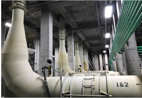
Photo: CSO Tunnel Pump Station
