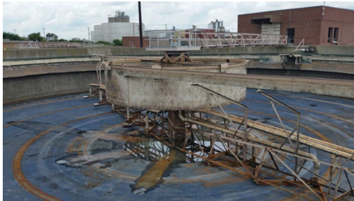
FPWWTF Wet Weather Clarifier
