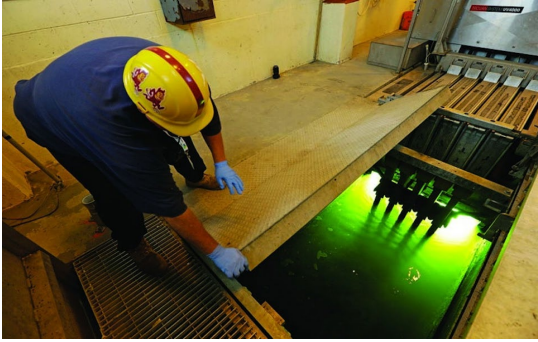
Photo: Bucklin Point UV Disinfection System
