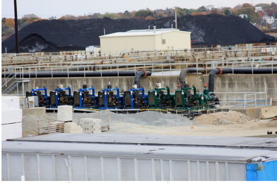
Photo: Aeration Tank Pumps
