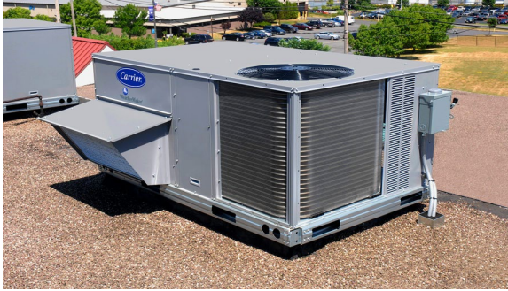
Photo: Rooftop Air Conditioner
