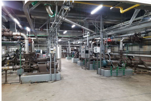
Photo: Primary Sludge Pump Station
