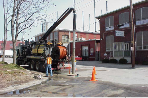
Photo: Interceptor Grit Removal
