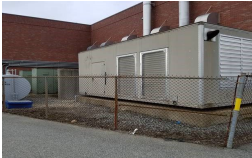
Photo: Field's Point Screw and Blower Generator
