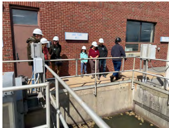
FP Supervisor Liam Walsh showing a group the grit tanks, part of preliminary treatment.
