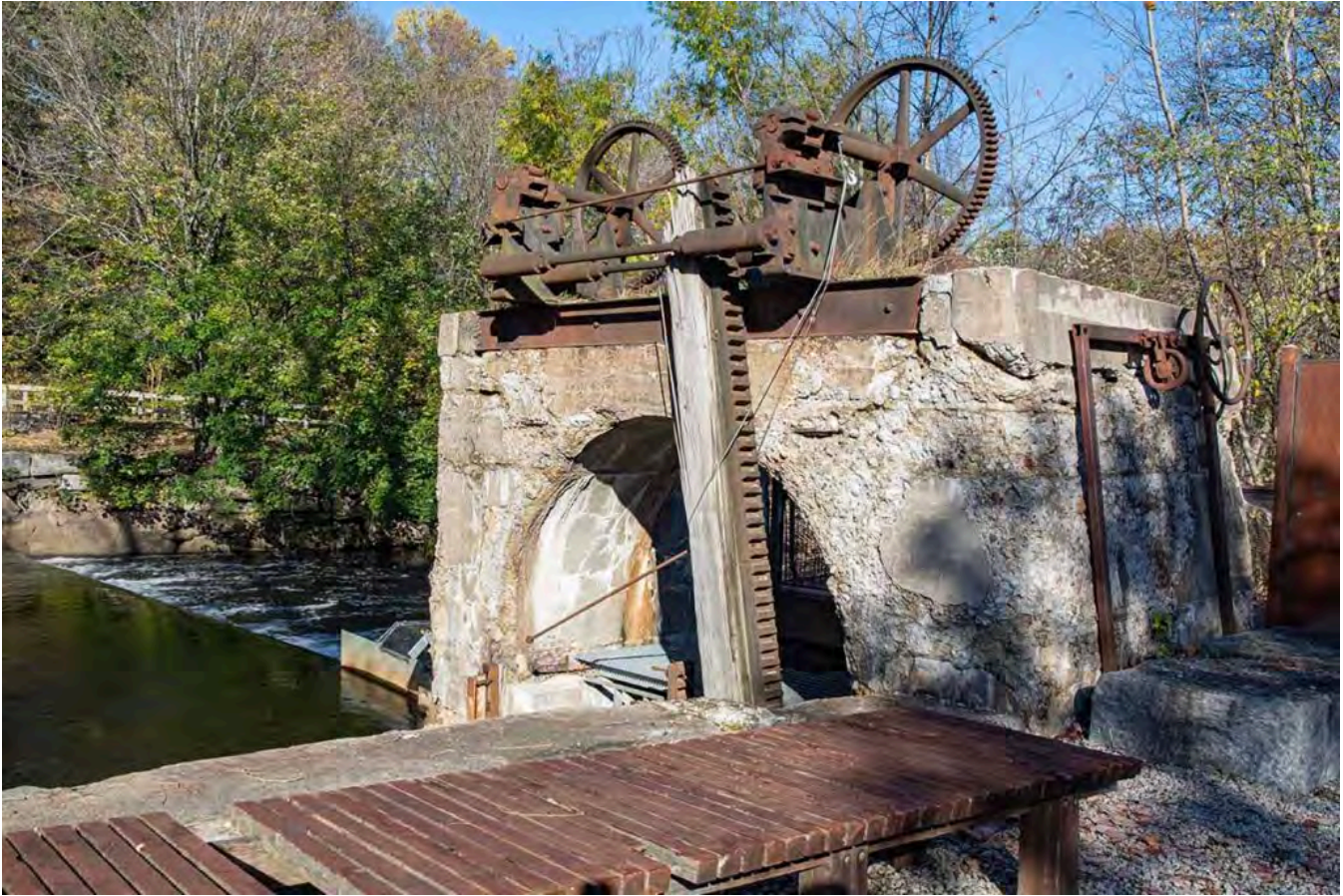
The remains of a sluiceway that once controlled the flow of the Woonasquatucket River.
