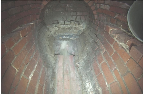
Photo: OF 056 Regulator on Vandewater Street
