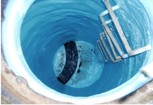
Photo: Flow Monitor
