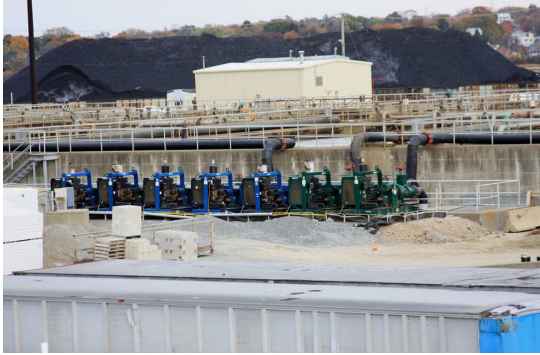
Photo: Aeration Tank Pumps
