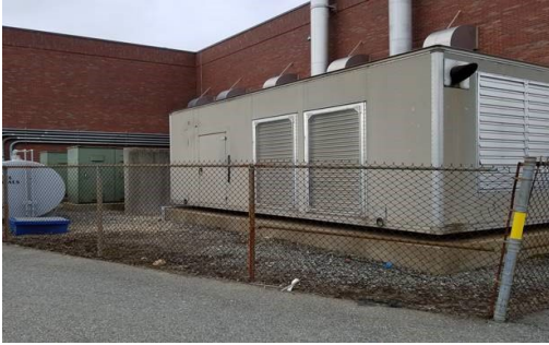
Photo: Field's Point Screw and Blower Generator
