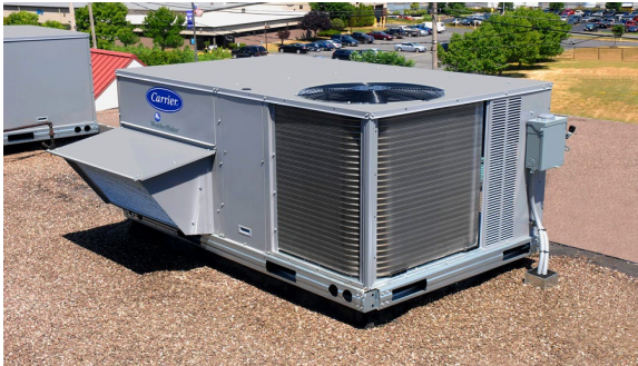
Photo: Rooftop Air Conditioner
