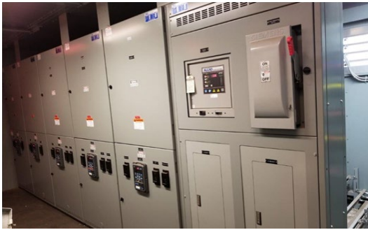
Photo: Field's Point Electrical Facility
